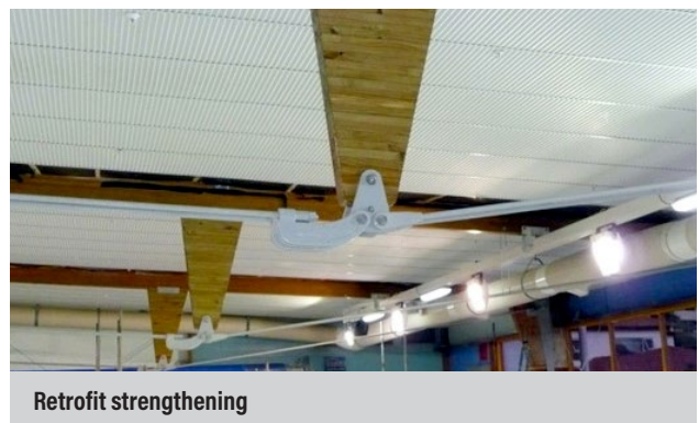
Wall Panel Tie-back
